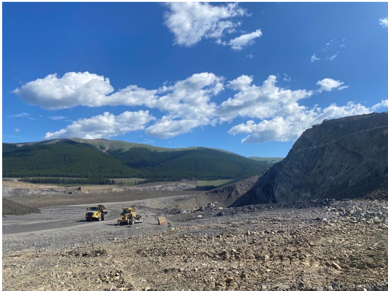
Backdropped by sensitive subalpine forests along the Eastern Slopes, heavy equipment works on the mammoth-task of coal mine reclamation. Photo © K. Halvorson.
