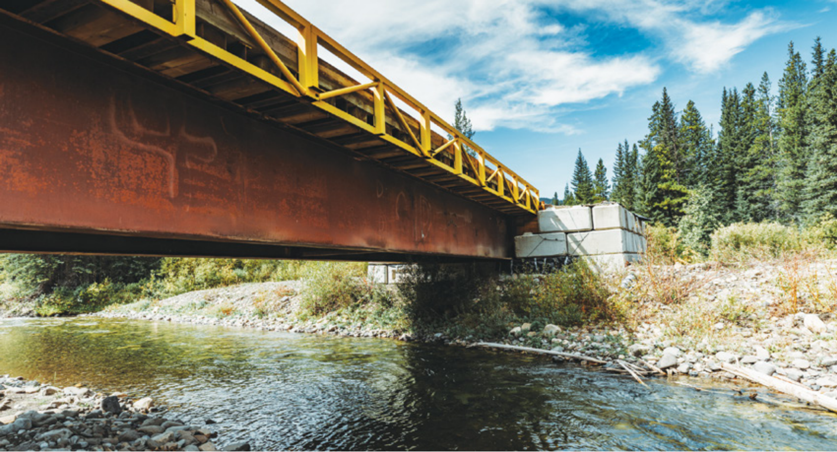
The bridge built over critical habitat for bull trout by Spray Lake Sawmills. Photo © A. Toner
