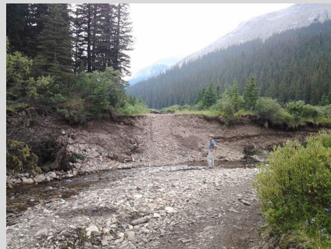
CAN water crossing Taken 2014-08-12 Severity: 5 L: 15m, W: 3m, D: 250cm
