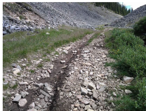
BTR damage site Taken 2012-07-19 Severity: 2
