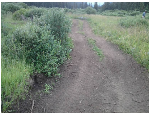
CAN damage site Taken 2014-08-12 Severity: 2 L: 40m, W: 3m, D: 40cm
