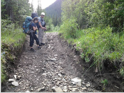
CAN damage site Taken 2012-07-18 Severity: 4 L: 30m, W: 3m, D:130cm
