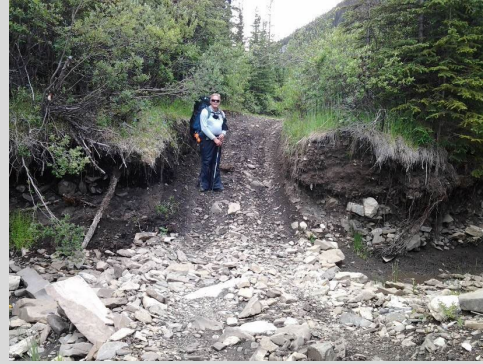
CAN damage site Taken 2016-07-06 Severity: 4 L: 15m, W: 3m, D: 120cm
