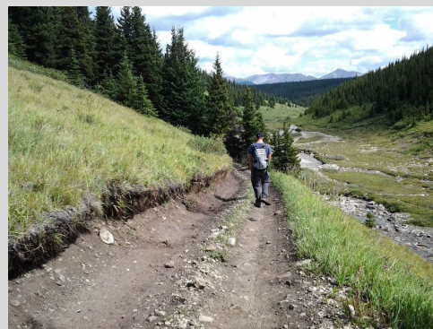
BTN damage site Taken 2016-08-04 Severity: 3 L: 76m, W: 1m, D: 60cm
