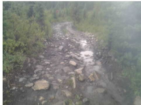
HUM damage site Taken 2016-08-03 Severity: 3 L: 50m, D: 25cm
