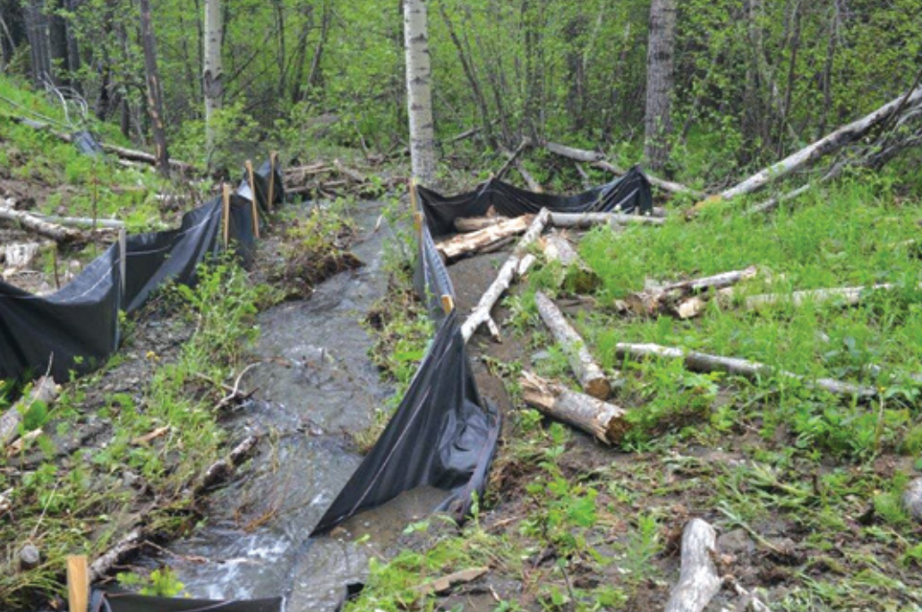
Ineffective effort to prevent excessive runoff from entering a tributary of Hidden Creek. PHOTO: © L. FITCH
