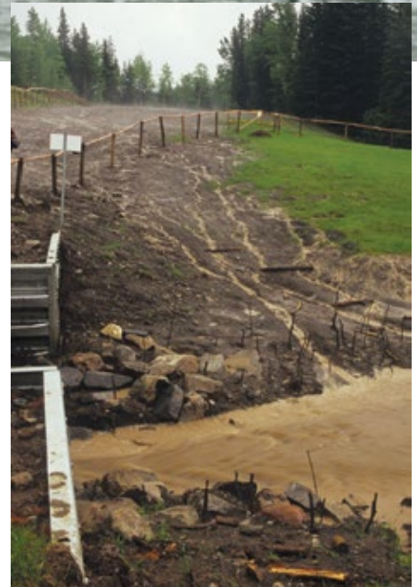
Poorly designed roads such as this one in the McLean Creek off-highway vehicle area send silt and sediment into streams to kill fish. PHOTO: © L. FITCH
