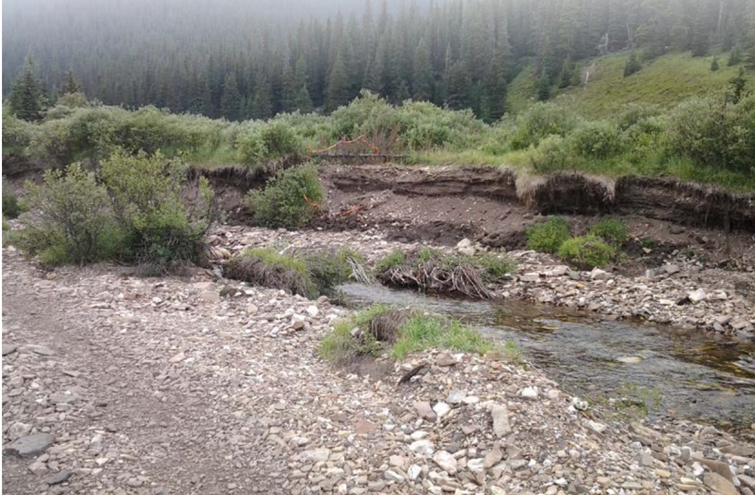
Fallen flagging shows where the bank has eroded further from last year and continues increasingly to undercut the trail. This creek is very much alive and is damaged significantly by infrastructure like OHV trails. PHOTO: © S. NICHOLS
