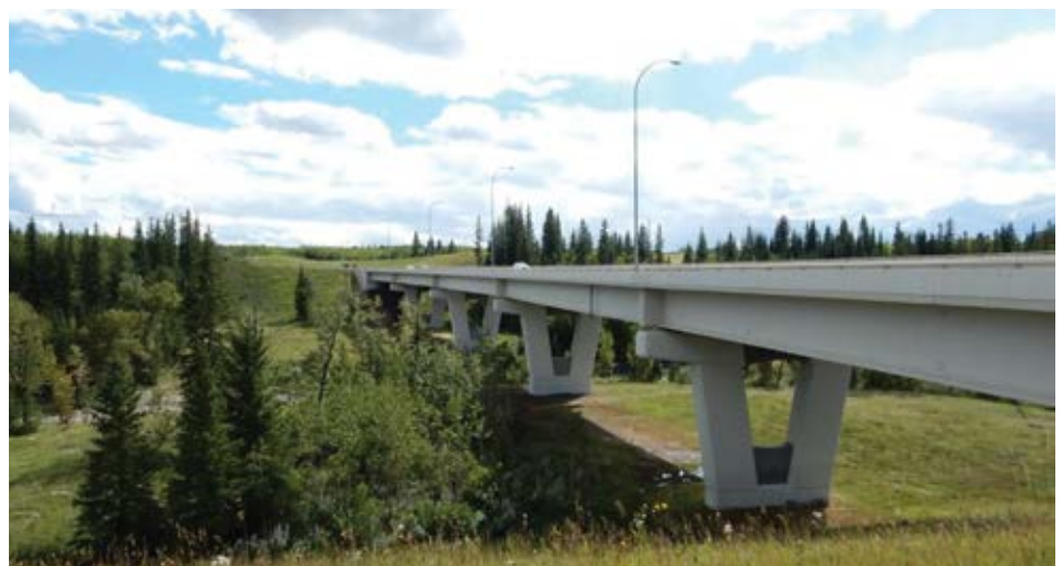
We know how to leave room for the river: the current 37th St. bridge across Fish Creek leaves a natural floodplain and wildlife corridor relatively intact. PHOTO: © E. MCMAHON
