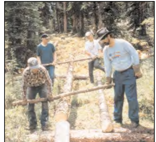
Volunteers lay the stringers for a corduroy bridge that was built over a sensitive wetland on the historic trail.
