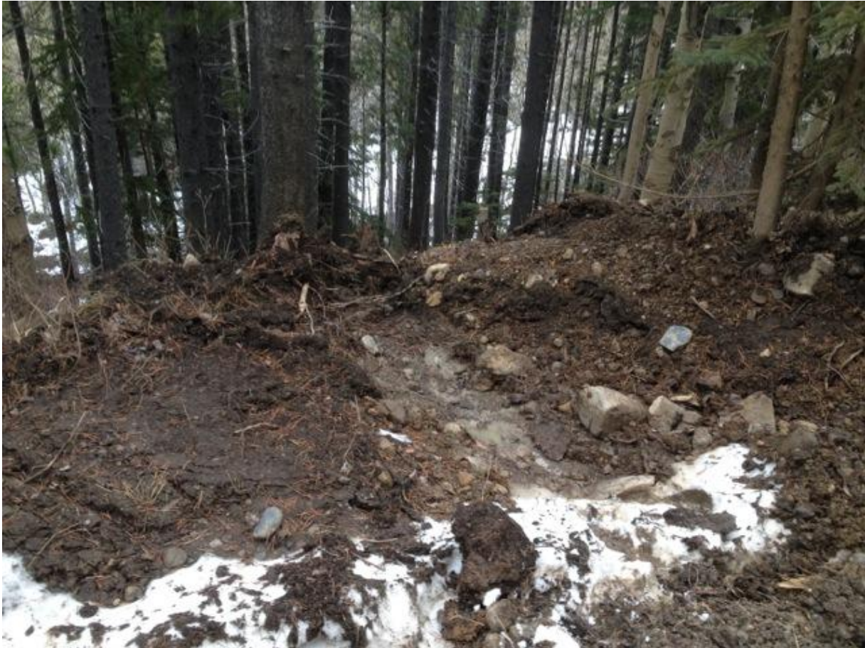
Inadequate mitigation measures along Canfor's haul road will result in slope erosion and sedimentation in Girardi Creek
