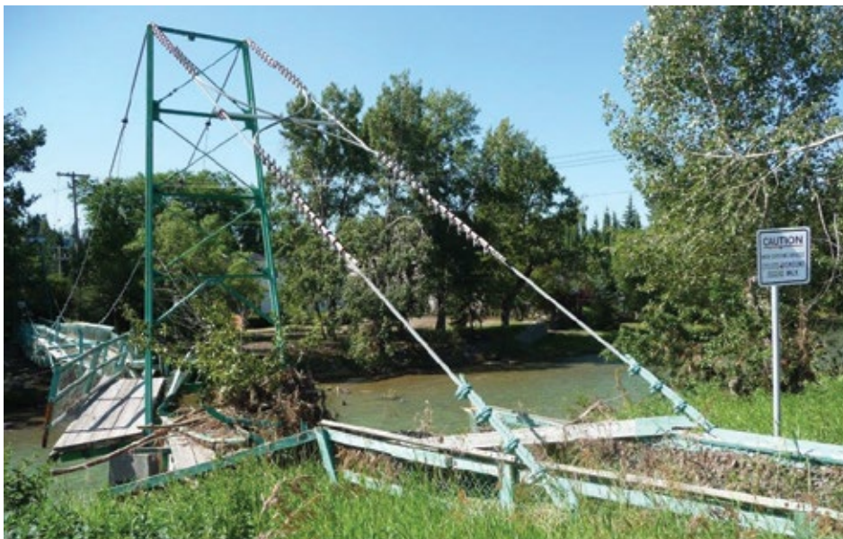
Elbow Park bridge after the Alberta Flood of 2013 PHOTO: © H. JULL
