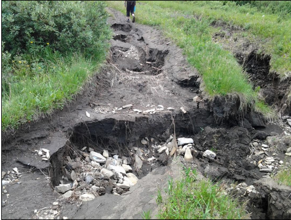
Figure 8. A section on CAN trail made impassable due to extreme erosion.
