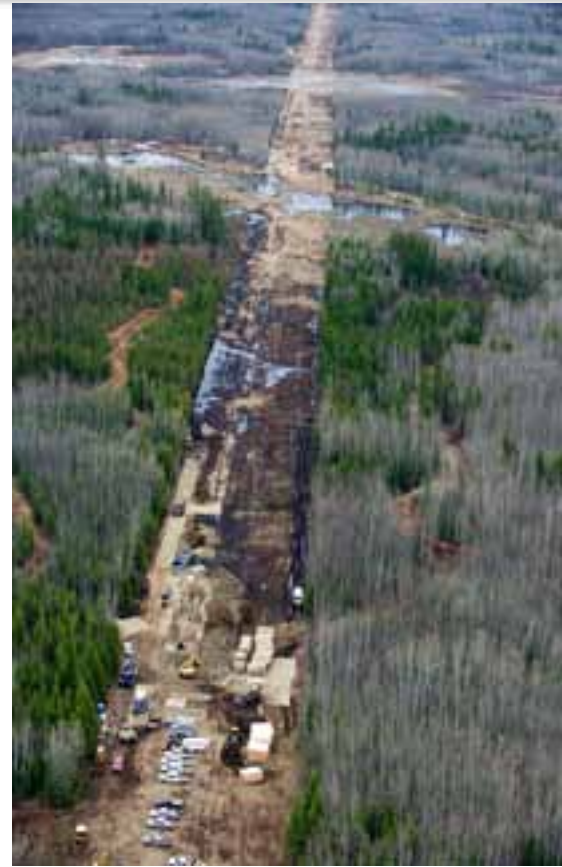
Crews work to clean up the Rainbow Pipeline oil spill, the worst Alberta oil spill in 35 years.
