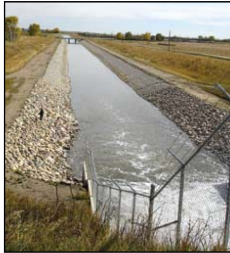
This irrigation canal is part of the Western Irrigation District's infrastructure to deliver water from the Bow River to more than 400 farms, 96,000 acres of land, and more than 12,000 people in four different communities.
