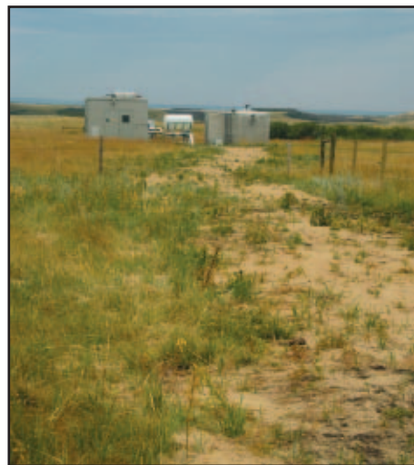
Canetic's well site in the Rumsey Natural Area showing a compressor and trenched in pipeline
