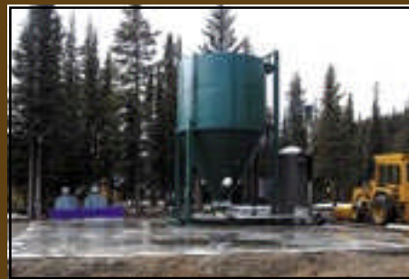
Fuel tanks, a concrete pad for a shop and a hopper that feeds fuel to an adjacent boiler at Panther River Adventures
