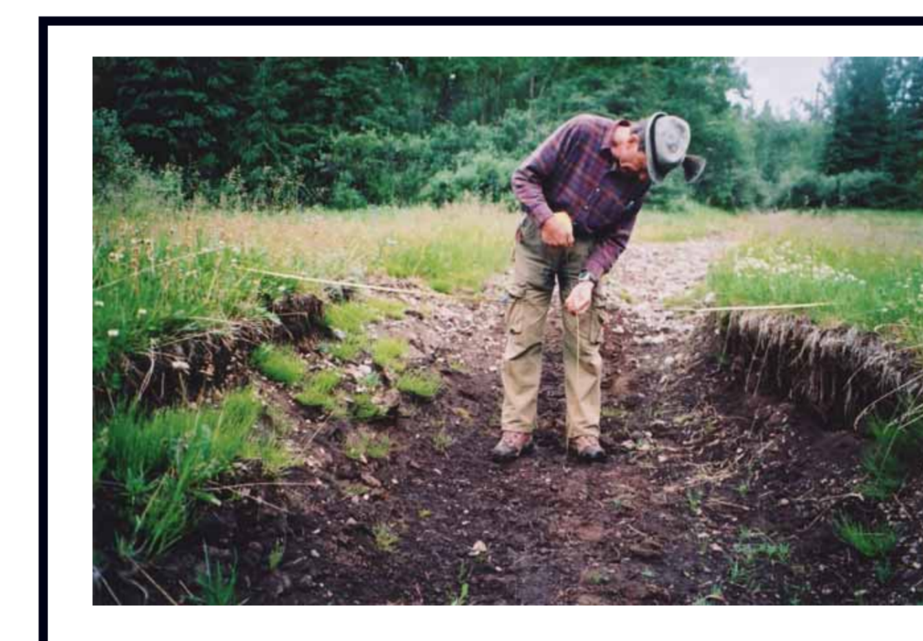
Measuring depth of severe rut along primary trail
