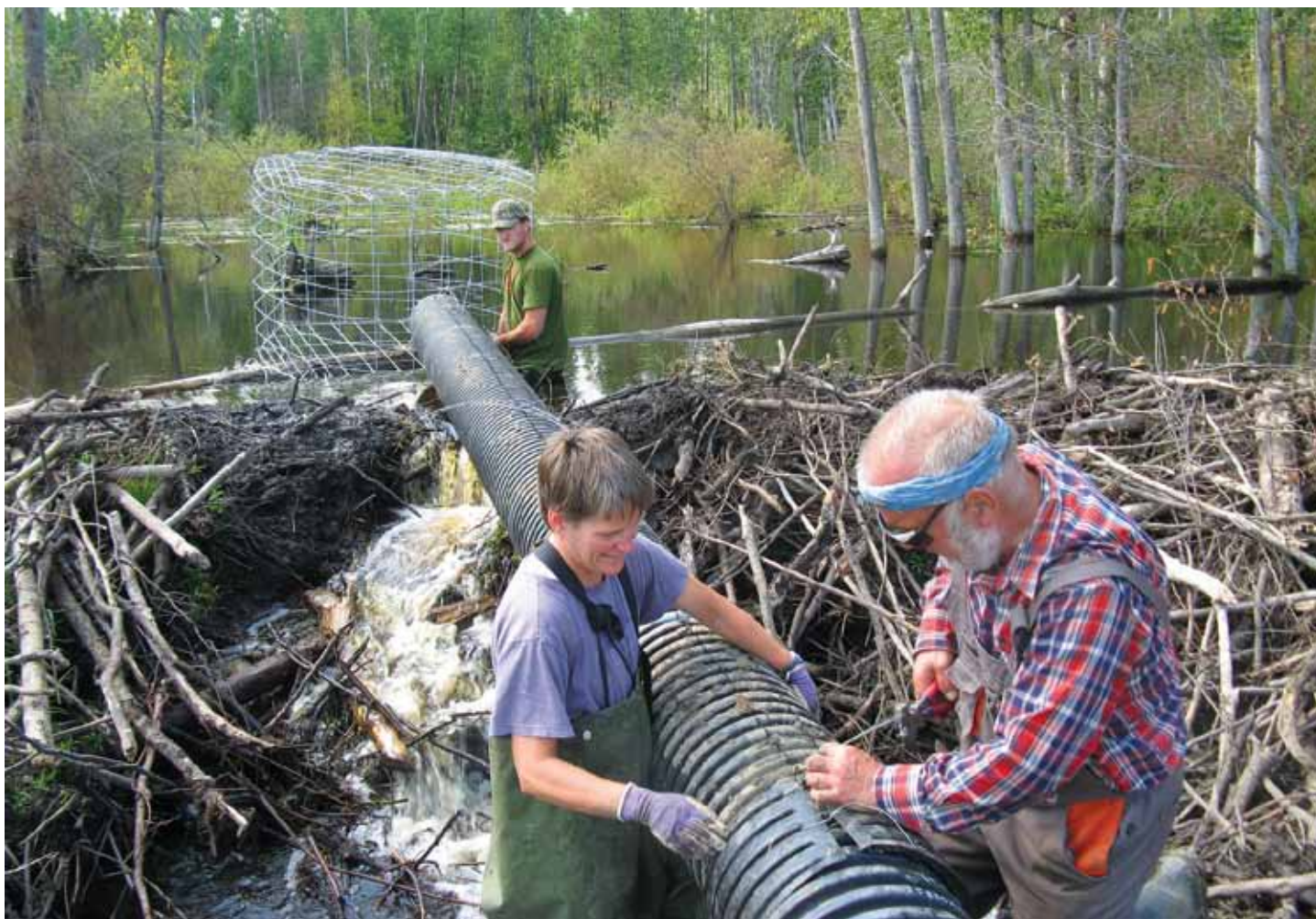
Installing a pond leveler to maintain water levels and prevent flooding of trails in the Cooking Lake/Blackfoot Provincial Recreation Area.
