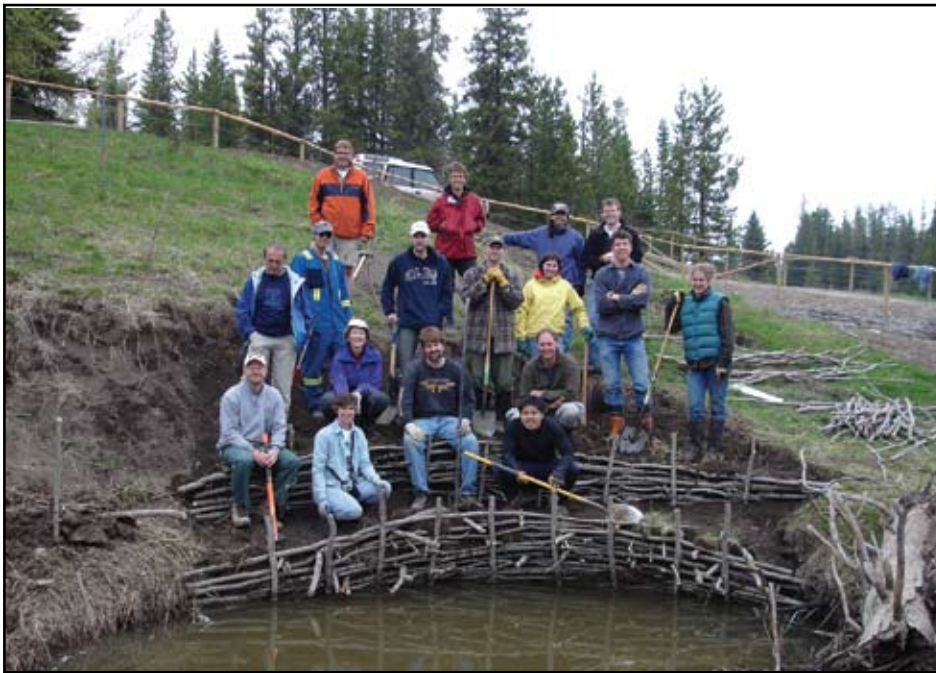
Stream bank stabilization using bioengineering – the Elbow River Watershed Partnership’s McLean Creek project west of Calgary, May 2007. Author is in second row, second from left. PHOTO: ELBOW RIVER WATERSHED PARTNERSHIP
