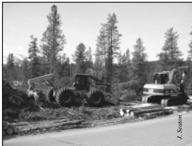
Skidder and steel-flanged felling machine used during the thinning operation in Jasper National Park during March 2004. Steel treads with flanges caused soil disturbance.
